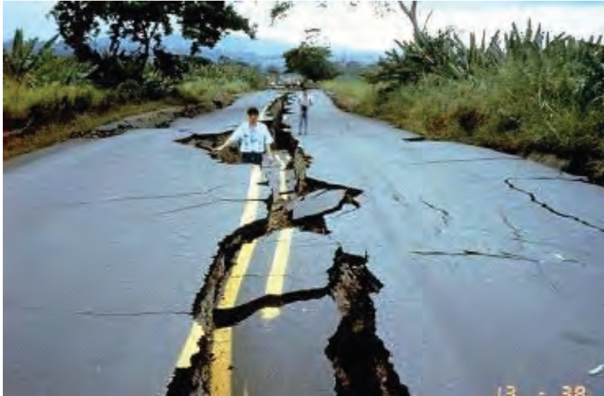
Figura I 26-2: Pavimento fracturado. (EERI) https://www.eeri.org/wp-content/uploads/costa_rica_1991_liquefaction.jpg
